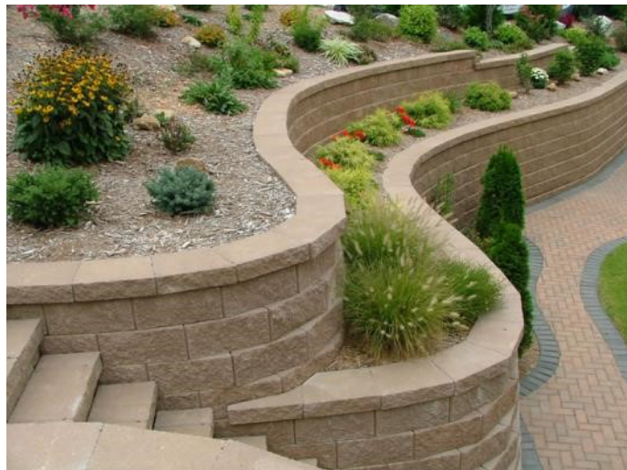
Figure 1113-C: This image illustrates a retaining wall that has been benched so that there is not a single, excessively tall, retaining wall.
