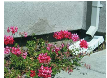
Figure 8-1: Disconnected downspouts drain to planted bio-filtration strips.
